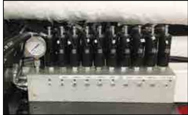
Fig 41 - Hydraulic valve bank
