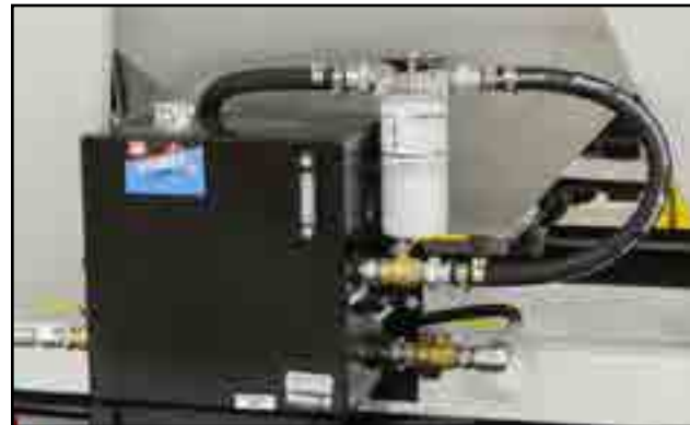
Fig 65 - Hydraulic oil reservoir and filter
