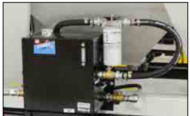
Fig 9 - Hydraulic oil reservoir and filter
