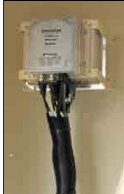
Fig 66 - Weigh Scale junction box
