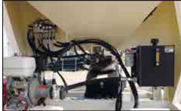
Fig 52 - Hydraulic oil reservoir and filter
