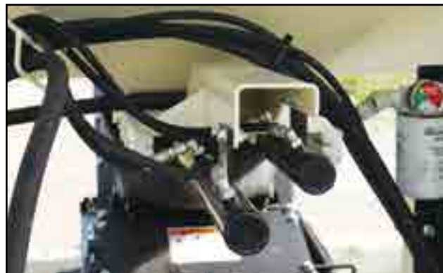
Fig 11 - Compartment slide gate cylinders
