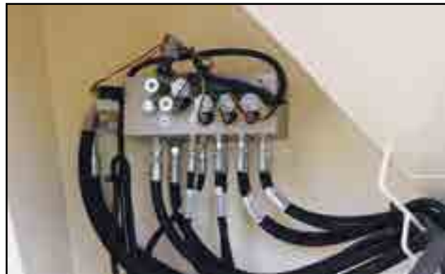
Fig 53 - Hydraulic valve manifold
