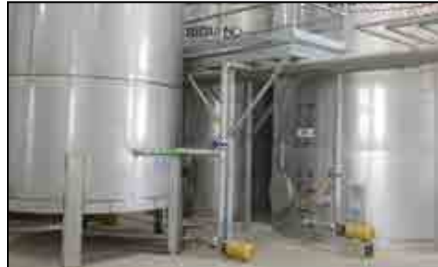
Fig 20 - Permanent fill and discharge system
