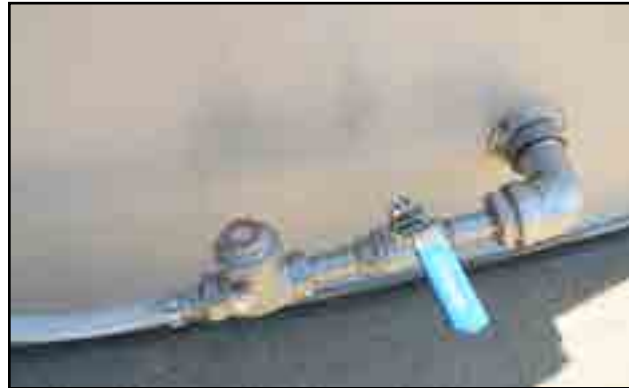
Fig 14 - Air intake pipe with valve
