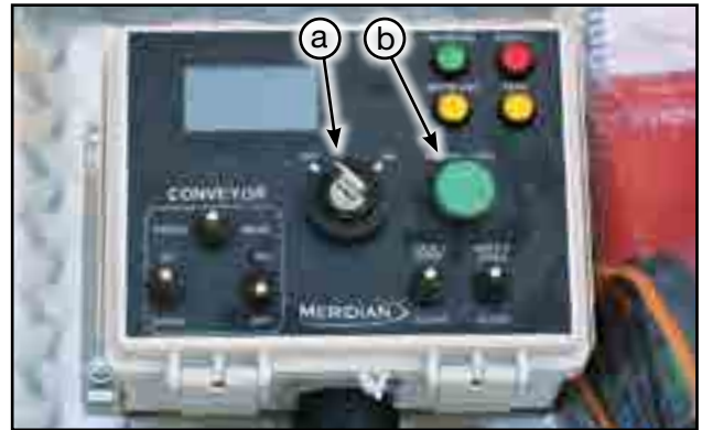
Fig 6 - Control panel inside box
