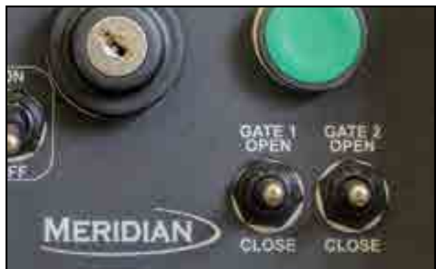
Fig 40 - Control box gate buttons
