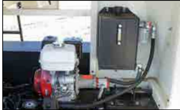
Fig 7 - Engine, hydraulic oil reservoir and filter
