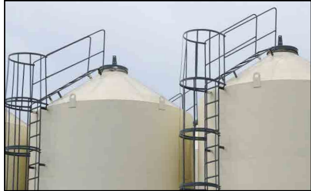
Fig 9 - Ladder cage and handrails
