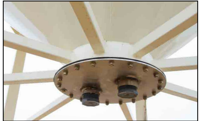
Fig 33 - Flange bottom on hopper
