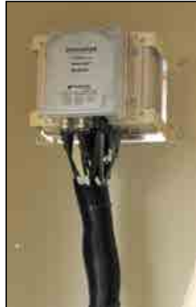
Fig 66 - Weigh Scale junction box
