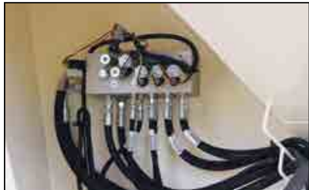
Fig 53 - Hydraulic valve manifold
