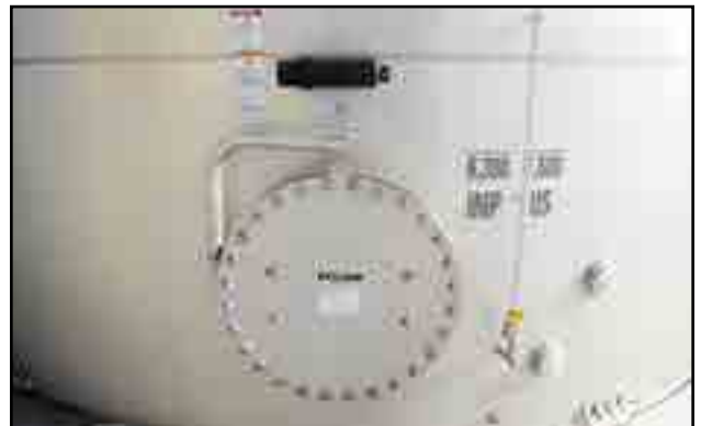
Fig 10 - Components on tank
