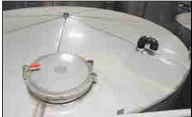
Fig 6 - Components at the top. Vent installed by customer
