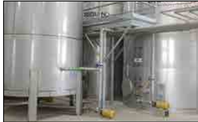
Fig 20 - Permanent fill and discharge system
