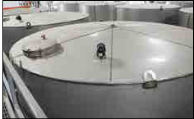
Fig 5 - Top of chemical tank
