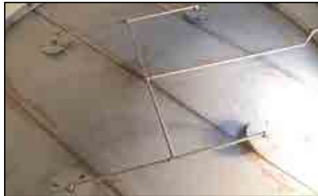
Fig 15 - Air injection diffusers
