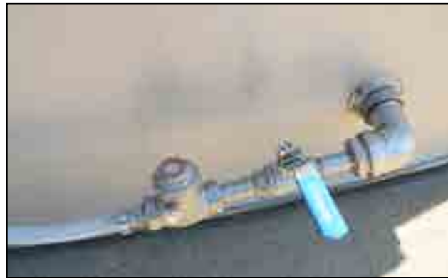
Fig 14 - Air intake pipe with valve
