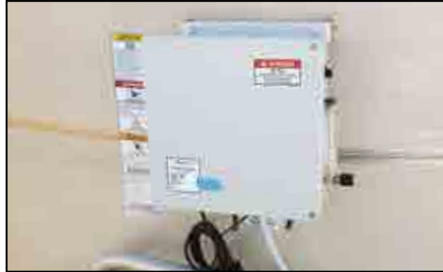
Fig 13 - Airmix liquid fluidizer control box
