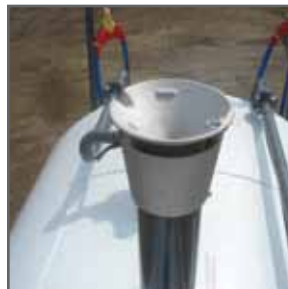
Vent Pipe 10,000L - 61,000L
